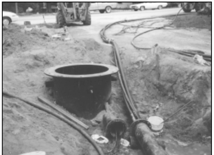
Remediation Well Head Manhole
